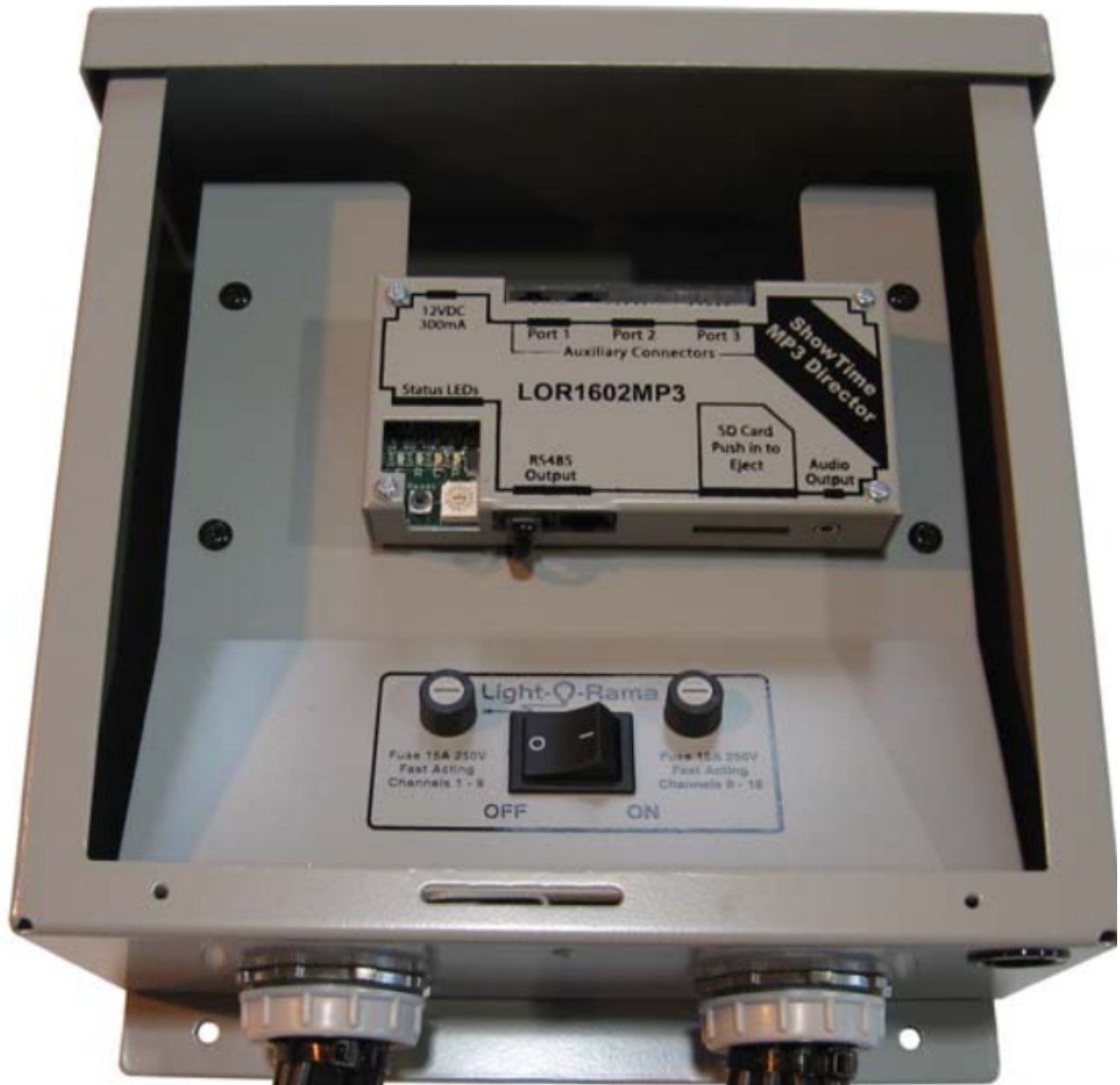
DC-MP3 as part of an LOR1602
